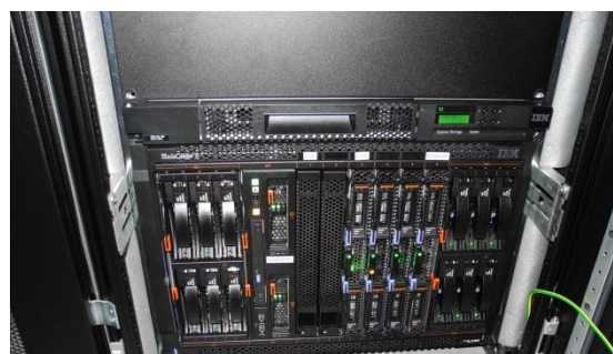
Modernste IBM Rack-Systeme
